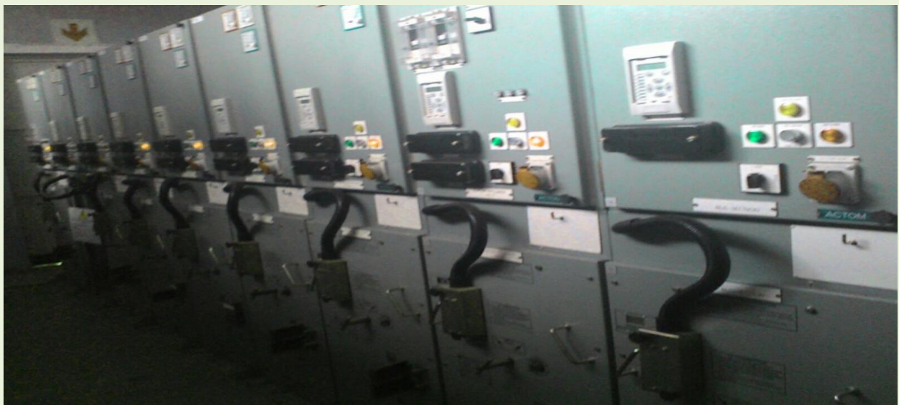
FIGURE:4 BELA-BELA SUB STATION
